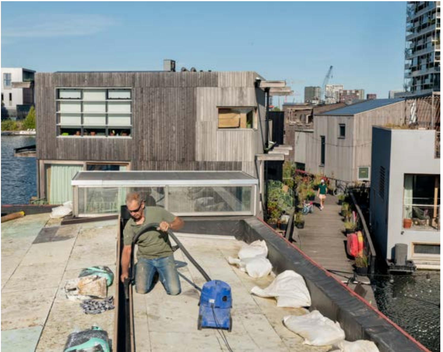
A resident doing maintenance on his roof in Schoonschip. It can be difficult to find contractors willing to work with the community's unusual requests. Max Pinckers for The New York Times
