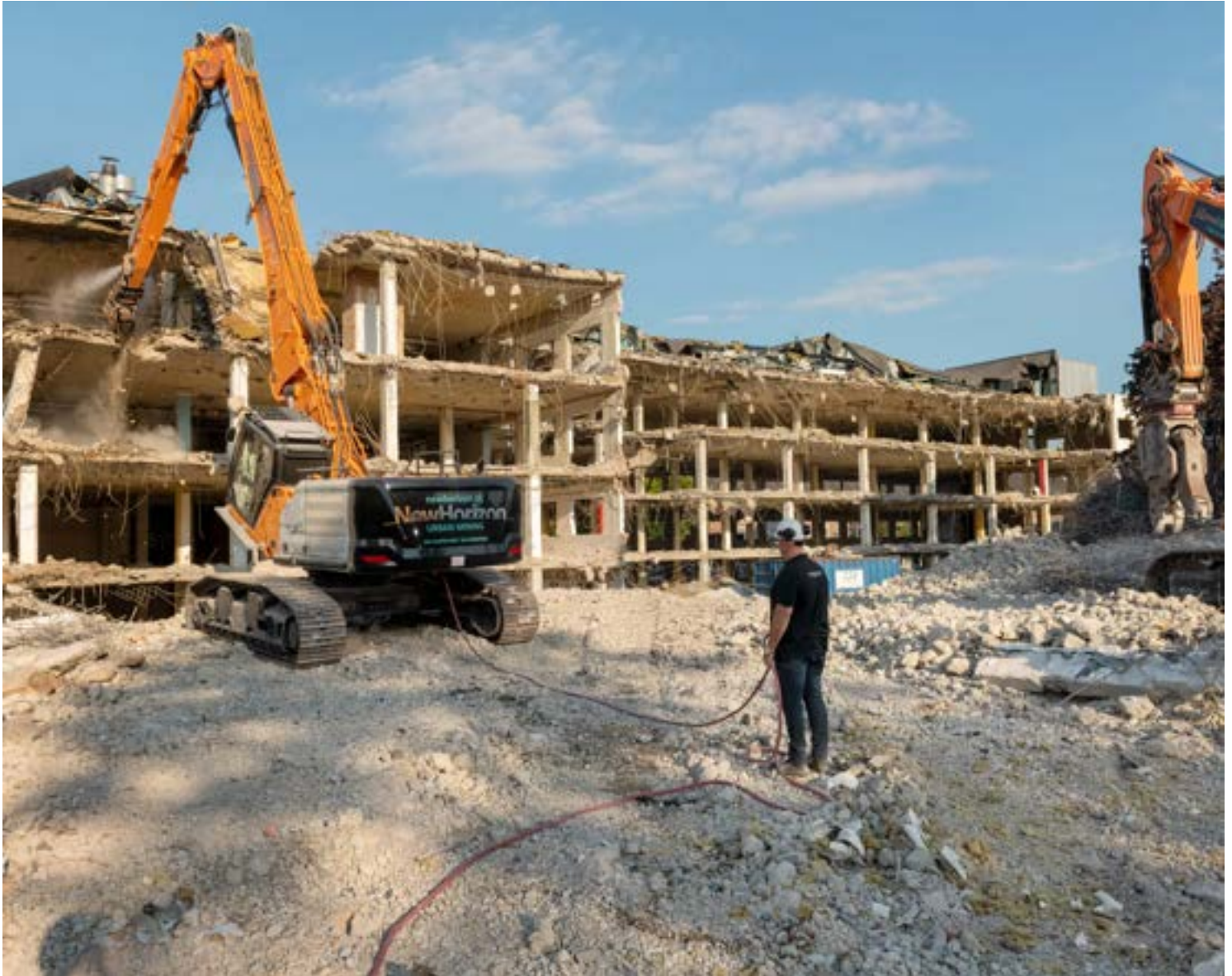
New Horizon taking down a hospital in Breda, a city in the Netherlands. Max Pinckers for The New York Times
